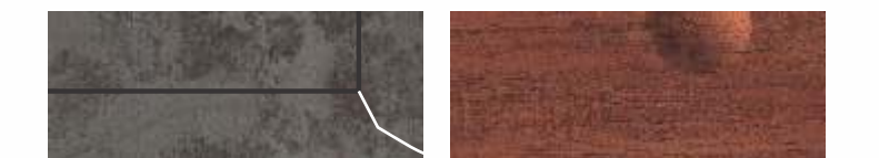
FOR CRACK ARISING OUT OF GROOVE CURRYING OR L SHAPE FOR AIR BUBBLES
