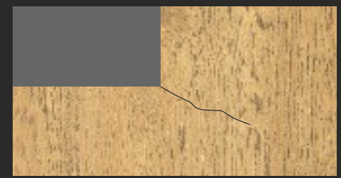
NO CLAIM WILL BE ENTERTAINED FOR CRACKING ARISING OUR OF GROOVE CURRYING OR L.SHAPE
