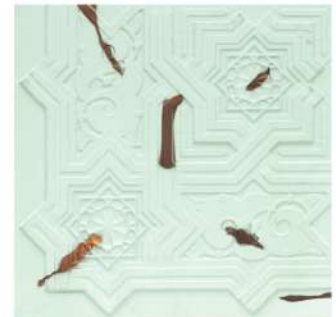
VC03 - Damaged Tin
