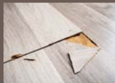
Cutting a laminated sheet at an angle of 90° leads to development of cracks in corner after pasting. Therefore it is advisable to void cutting at an angle of 90°.
